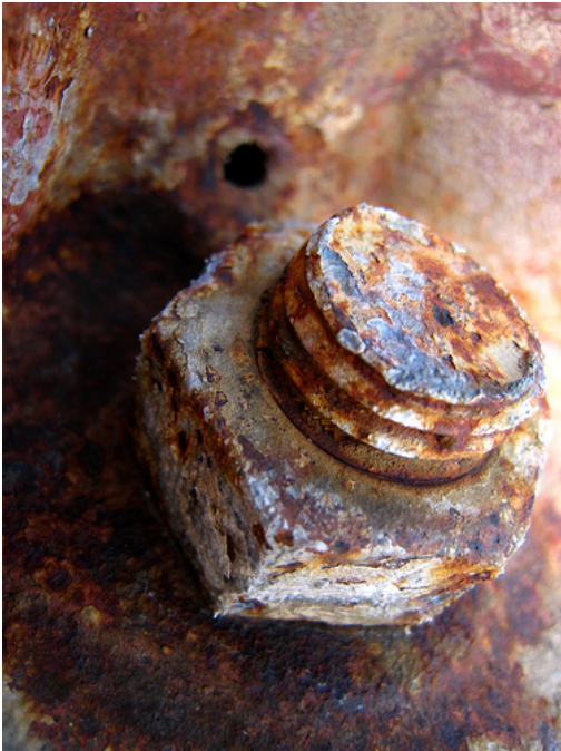
Florida, USA - failure of coating after 6 months
